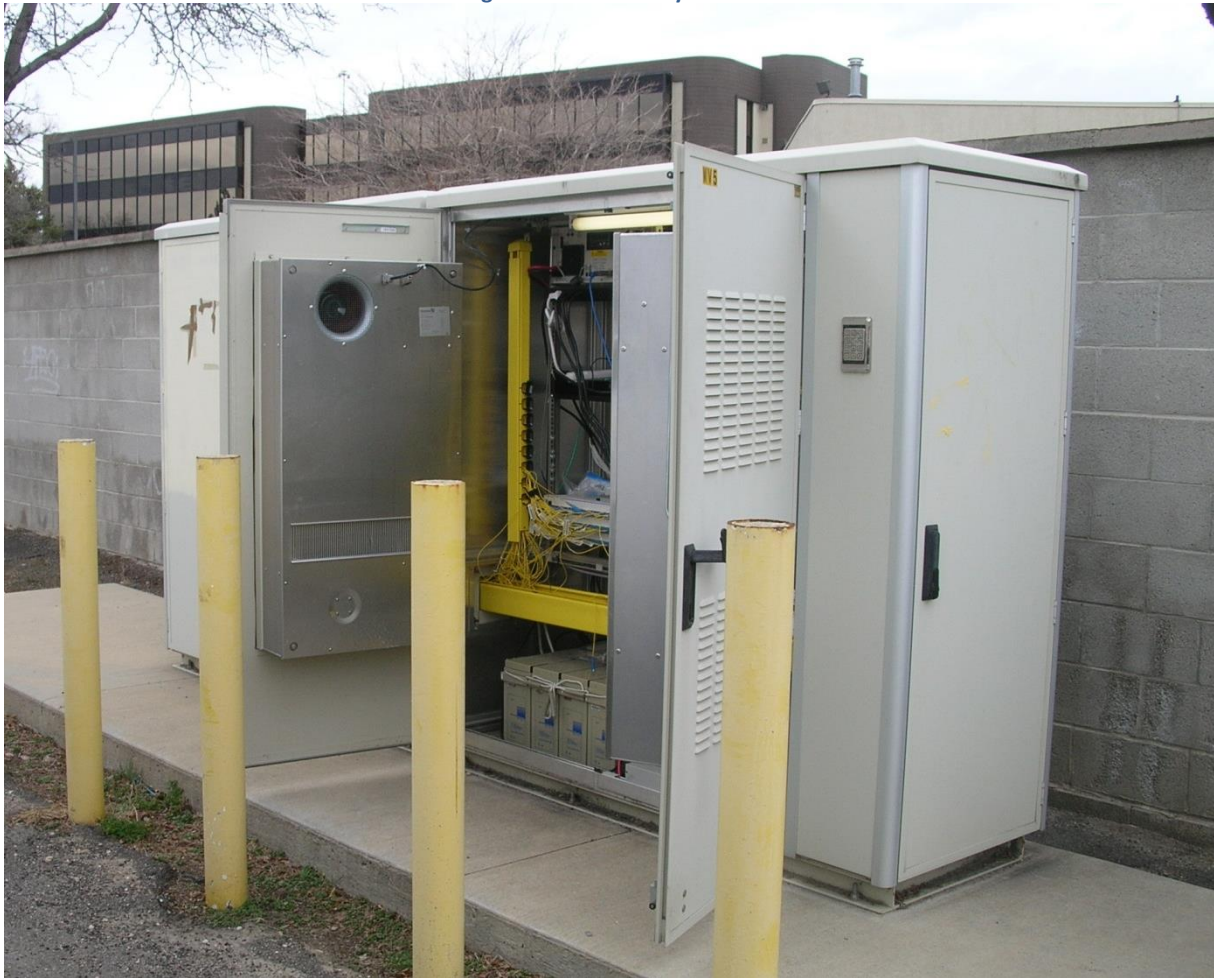
Figure 10: Hub Facility in Cabinet
