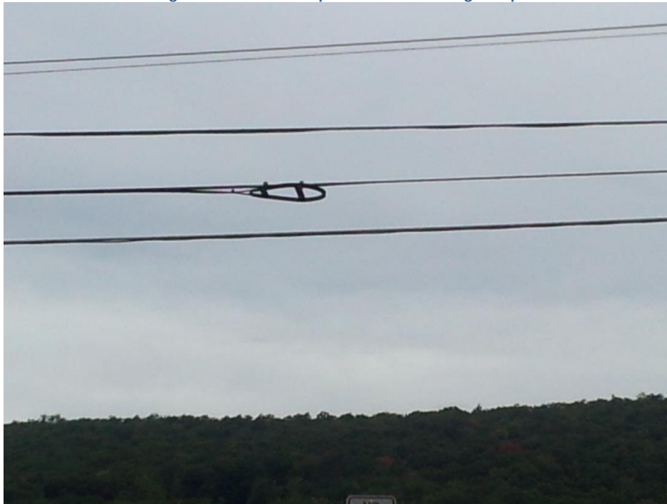
Figure 4: Aerial Fiber Optic Cable with Storage Loop
